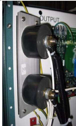
Figure 35: Output Lightning Arrestors
